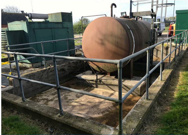
The main diesel bund prior to installation
